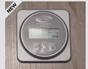
Battery digital display monitors battery statistics like amp-hours consumed, state of charge, and voltage.
