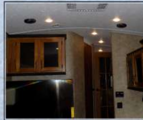
Eco-Friendly LED Interior/ Exterior Lighting
